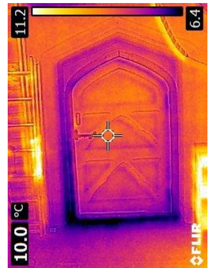
Photo 7 - West door - dark area at base of door indicate cold air blowing in
