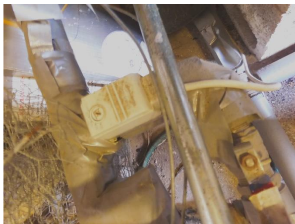
Photo 2 - Faulty pipework sensor next to boiler
