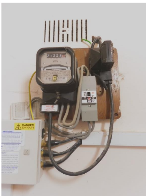
Photo 4 - Existing incoming 100A single phase supply
